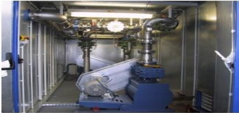
Gambar 2.9 Gas Blower (sumber : Horacio Terraza, 2009)
