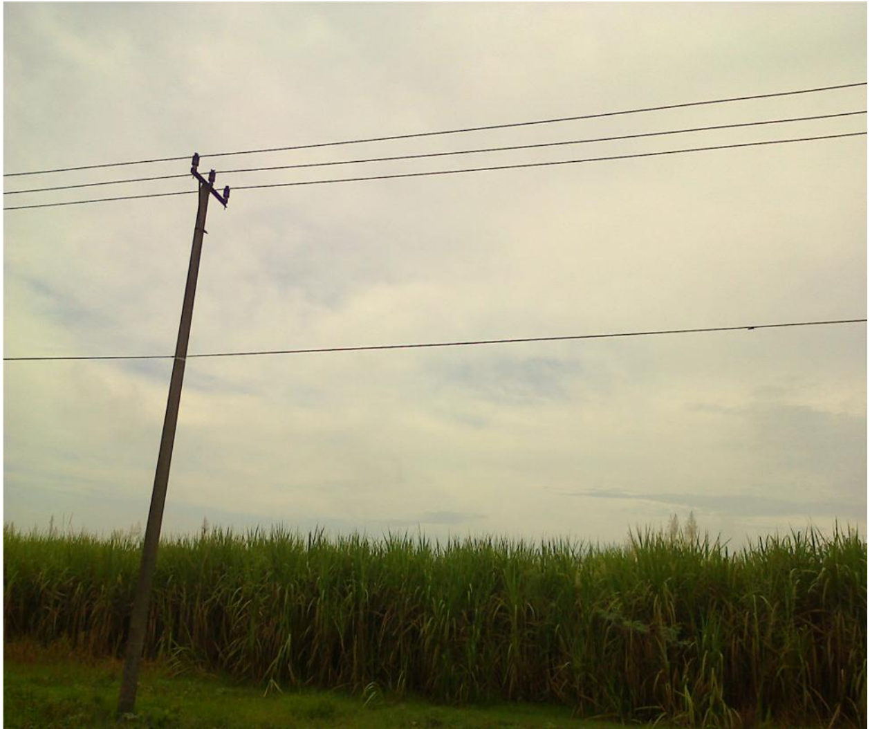
Keterangan: Tiang Listrik di PT. Sugar Group Companies (SGC)
