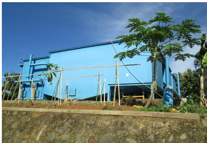
Gambar 2.20 Water Treatment Plant (WTP)
