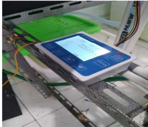
Gambar 3. 6 Water flow meter
