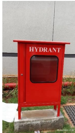
Gambar 3. 36 Hydrant Box Outdoor
