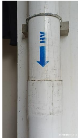
Gambar 3. 42 Pipa Air Hujan
