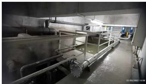
Gambar 3. 32 Sewage Treatment Plant (STP)
