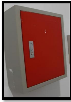
Gambar 3.32 Terminal Box Fire Alarm
