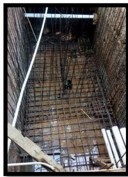
Gambar 3.41 ground water tank (GWT)
