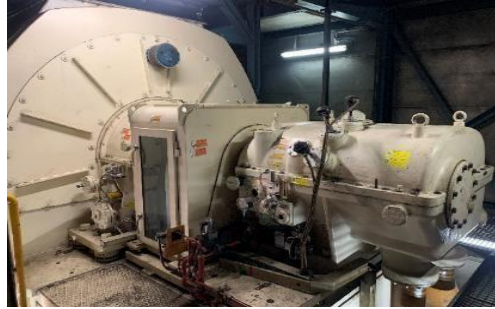
Gambar 2. 8 Main Oil Pump pada Lube Oil System
