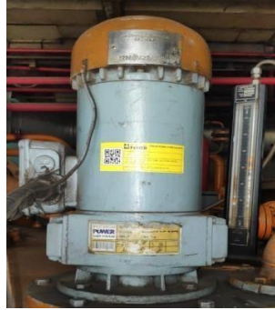
Gambar 2. 10 Emergency Oil Pump pada Lube Oil System
