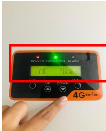
Gambar 3.14 LED Indicator PV Inverter
