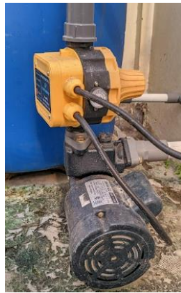
Gambar 2.12. Water Jet Pump dan Automatic Pump Control
