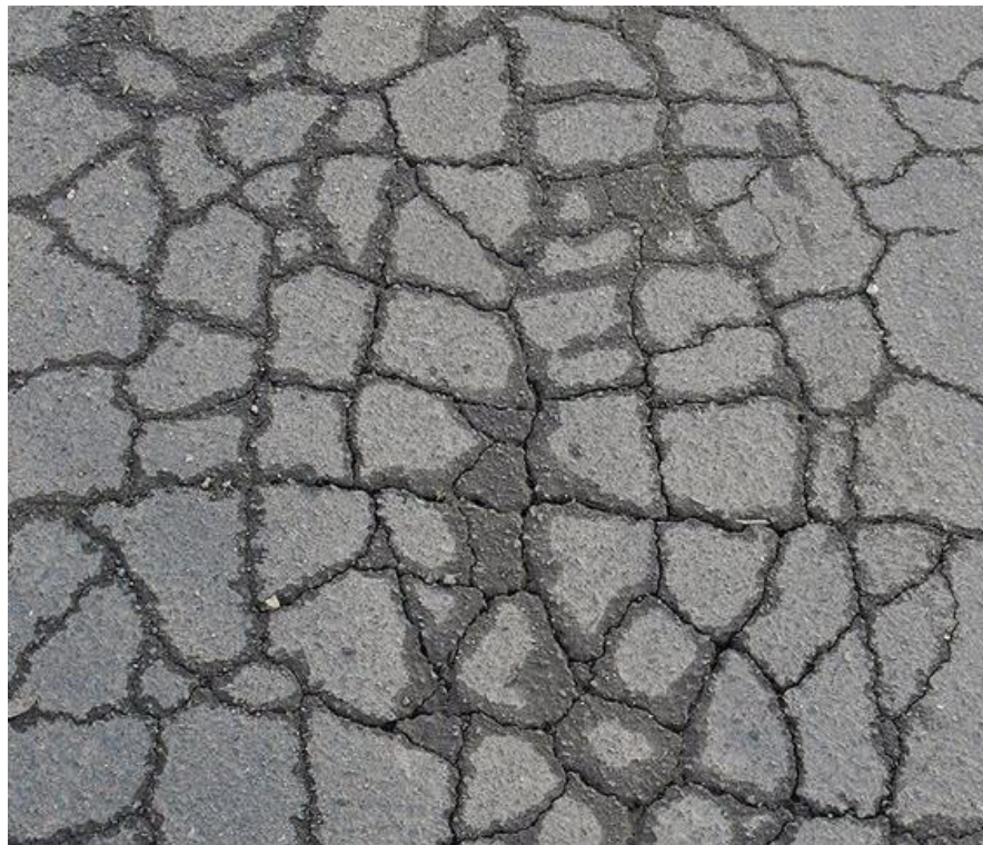
Gambar 2. Alligator Crack (Olahan Pribadi).
