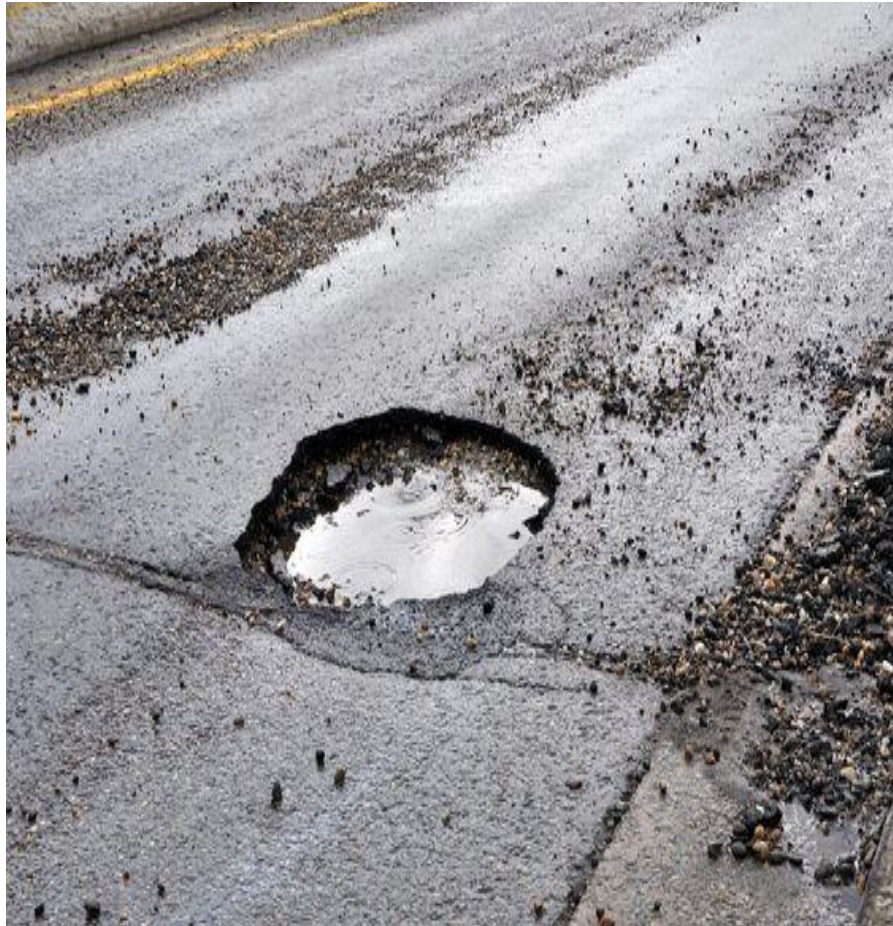
Gambar 5. Potholes (Jiang et al. , 2023)
