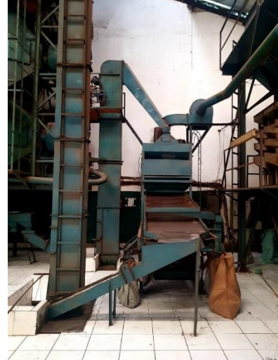
8. Elevator, Grader Drying oven
