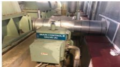
Gambar 2.9 Main Control Valve
