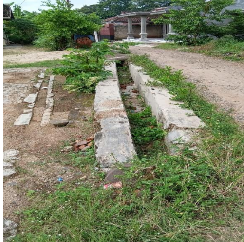
Gambar 12. Prasarana jaringan drainase
